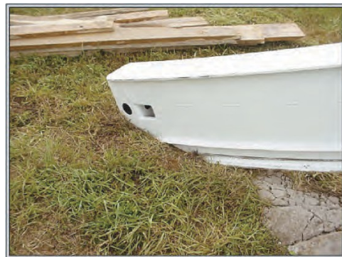
Figure 7 Punch through accident because of soil conditions
