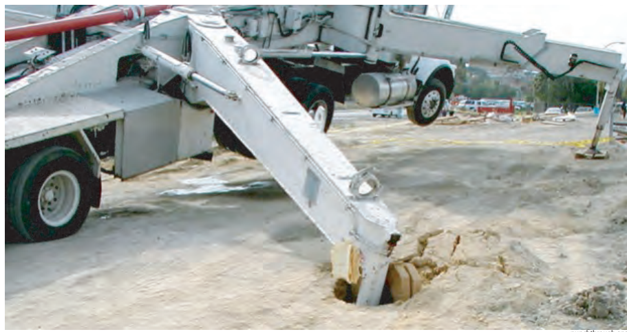
Figure 14 Hidden voids cause accidents
