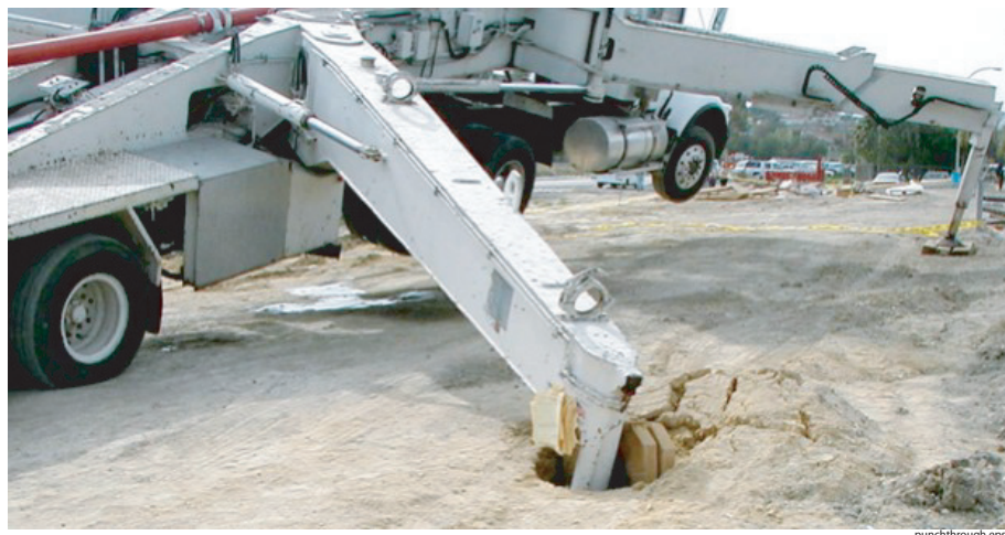
Figure 14 Hidden voids cause accidents
